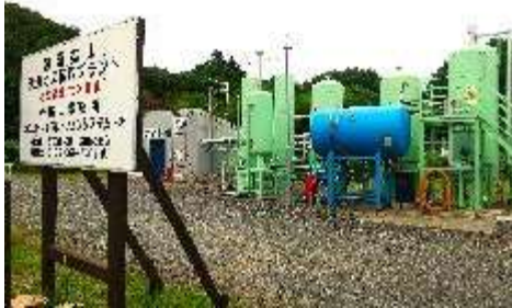
Natural gas extraction plant
